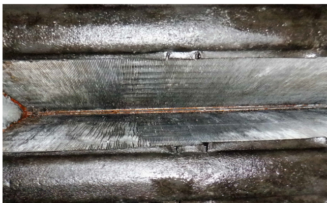
Very dirty AC coils. AC coils, blower, ducting must be clean for mold sensitive people
