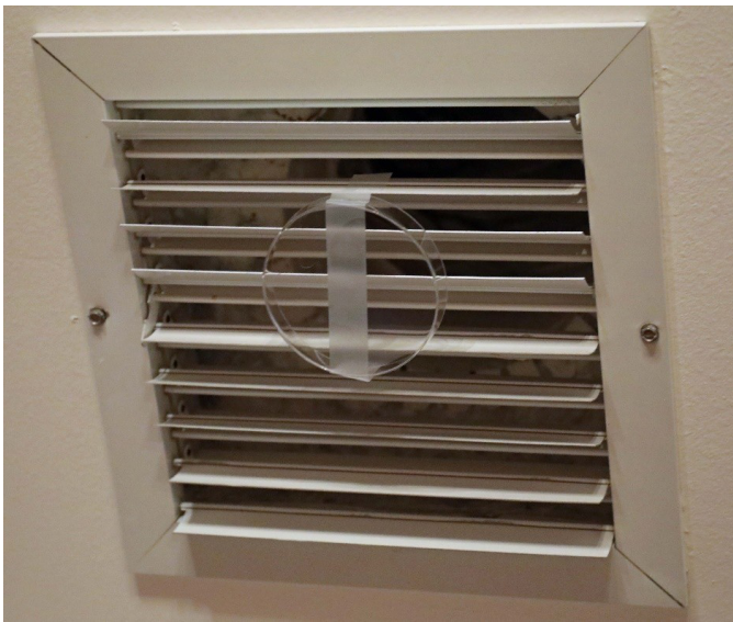
Tape petri dish to grill to check for mold spores coming from AC and ducting.
