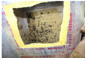
AC supply plenum (fiberglass box above the AC) is full of live mold.
