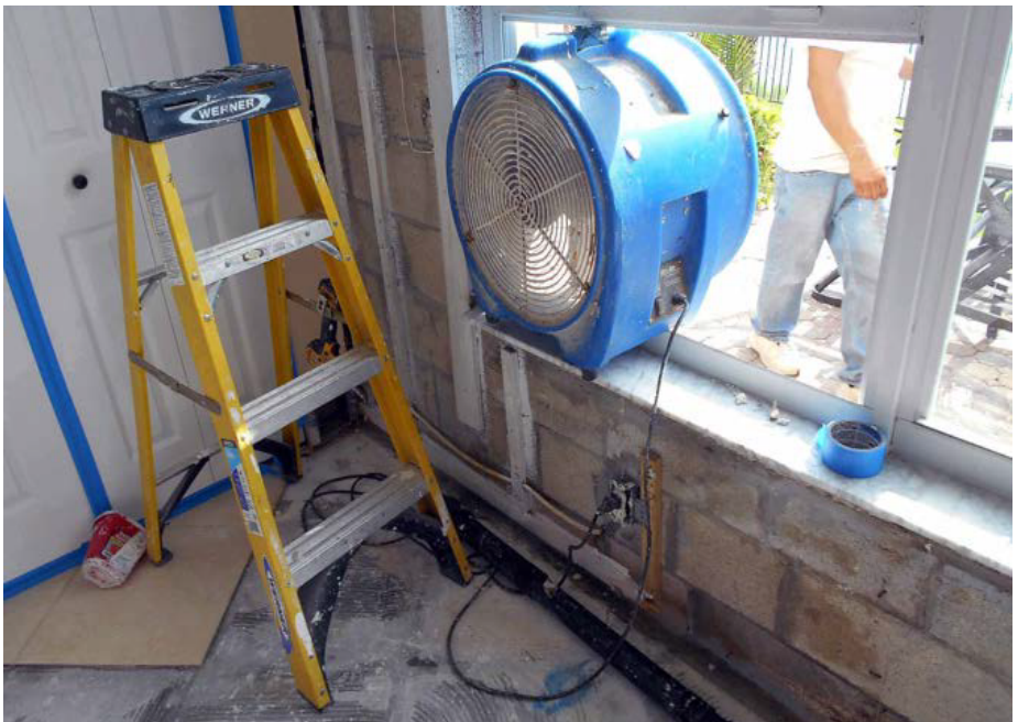
Axial fan in window okay if work is under or around window. Position fan blowing out of course to exhaust dusts and mold released by demolition outdoors.
